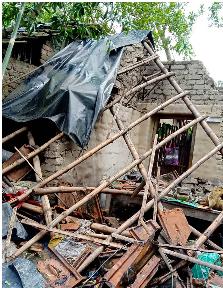
Damage to a home from Cyclone Bulbul, West Bengal, India, 2019. PHOTO: DEBABRAT PATRA/ACTIONAID
